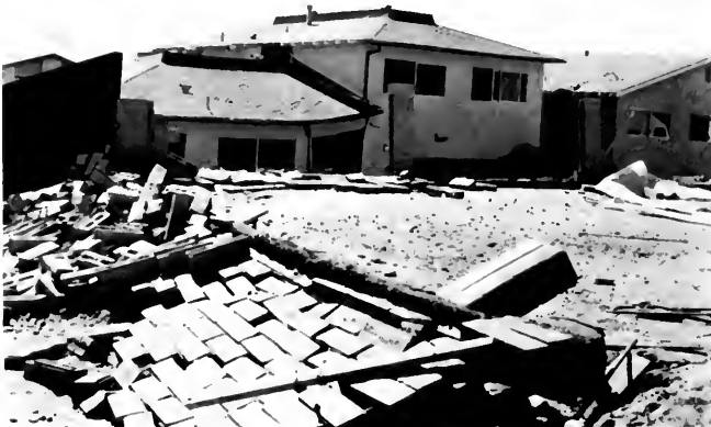
Photo 16. Example of collapse of single-story unit and pull-away between single and two-story portions (Almetz Street-Aldergrove Avenue). Courtesy of the City of Los Angeles Department of Building and Safety.
